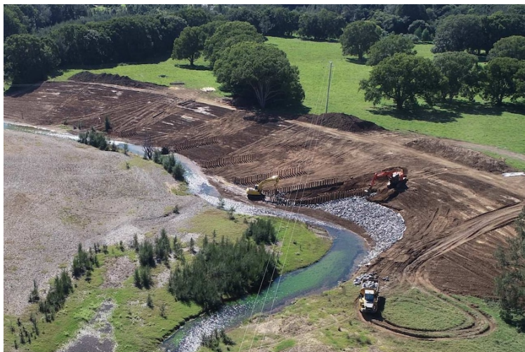
The river repair site during restoration at Kenilworth in 2019.(Supplied: Burnett Mary Regional Group)
